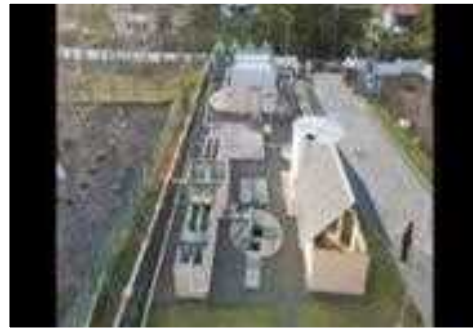
1 MLD CSTP at Padanappalam, Kannur
