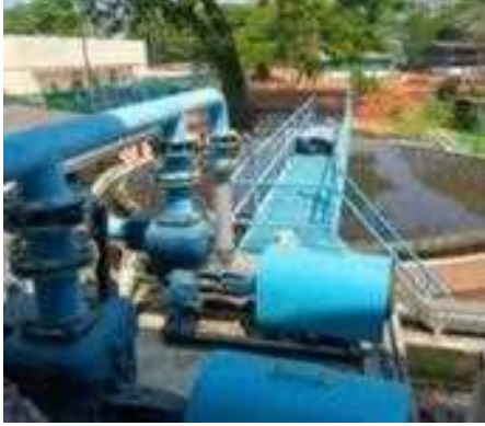
500 KLD STP at Kozhikode medical College
